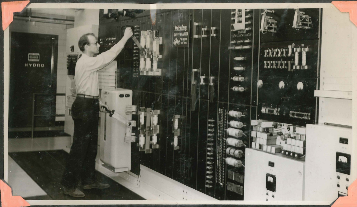
POWER SUPPLY FOR THE EQUIPMENT CONTAINED IN THE CENTRAL OFFICE IS SUPPLIED FROM THIS THREE SECTION RECTIFIER PANEL IN THE BASEMENT OF THE BUILDING. THE PANEL IS ALSO USED TO RE-CHARGE BANKS OF BATTERIES.
