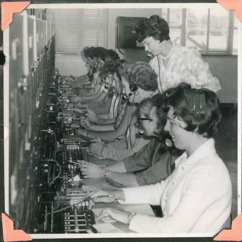
CHIEF OPERATOR AT THE TRAFFIC DEPARTMENT, MRS. E. DEMERY, GIVES ADVICE TO OPERATORS ON THE SWITCHBOARD. OPERATORS NO LONGER USE DIALS TO MAKE A CALL, INSTEAD NUMBERS ARE "KEY PULSED" WITH BUTTONS MARKED IN THE SAME WAY AS THE DIAL ON THE TELEPHONES
