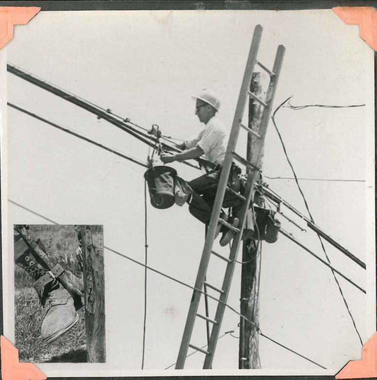
SECTIONS OF THE NEW CABLE BEING INSTALLED ON GARRISON ROAD ARE SPLICED TOGETHER BY SPLICER KEN GRIMWOOD. THERE ARE 400 PAIRS OF WIRES IN THIS CABLE. SPURS (INSET) ATTACHED TO LINEMAN'S BOOTS, SHOW METHOD USED FOR MEN TO CLIMB.
